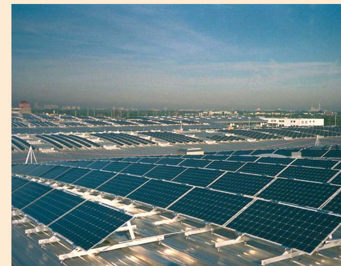
PV System Munich Trade Fair Centre
