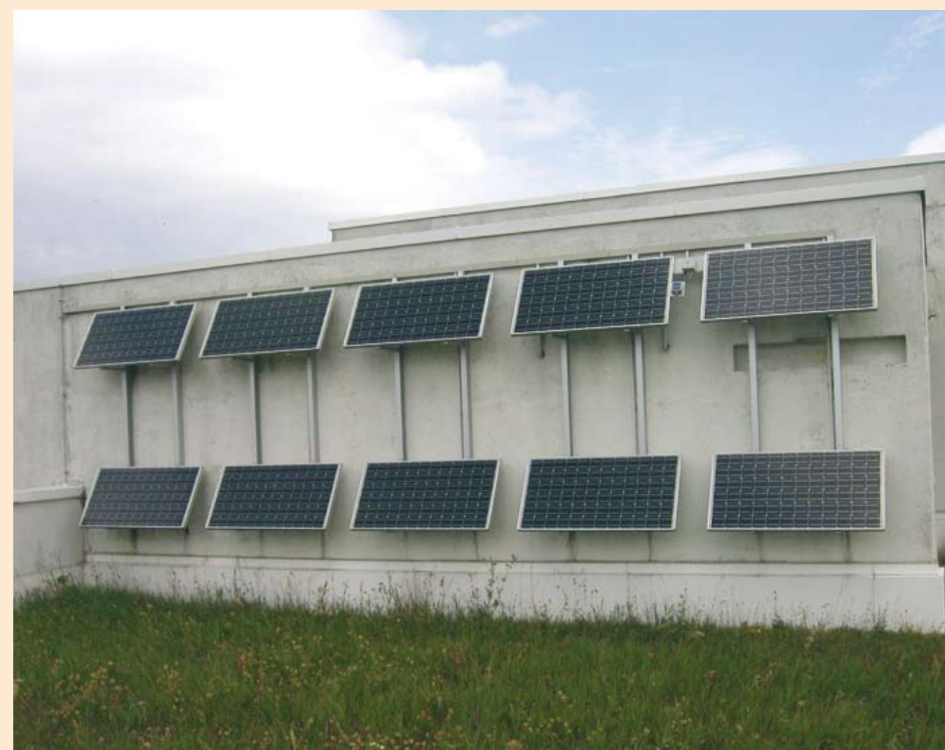
"Sun at School" PV Plant in Munich
