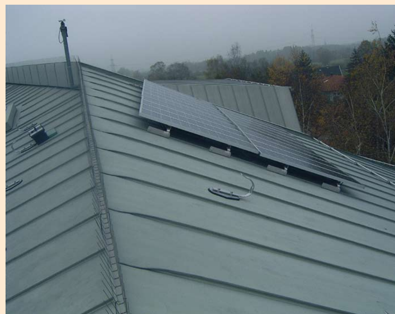
"Sun at School" PV Plant in Gröbenzell near Munich
