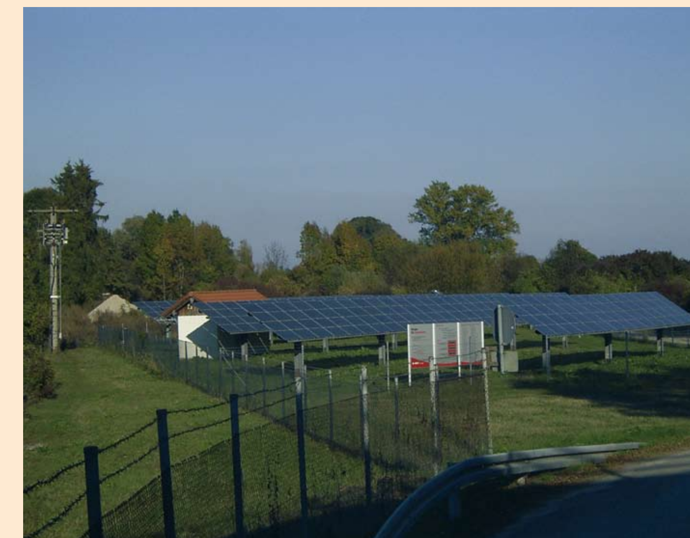
"Citizens for Solar Power" PV Plant in Unterföhring near Munich
