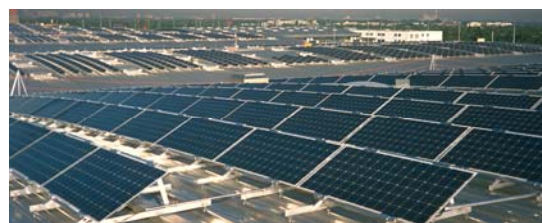
Figure 1: 1 kW p school PV system installed in 1995 (above), 50 kW p system (1994 - middle), 1 MW p PV system Munich Trade Fair centre (1997- below)
