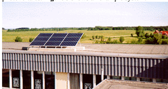
Figure 3: SONNEonline - 1.0 kW PV system of a grammar school in Samtens in the north of Germany
