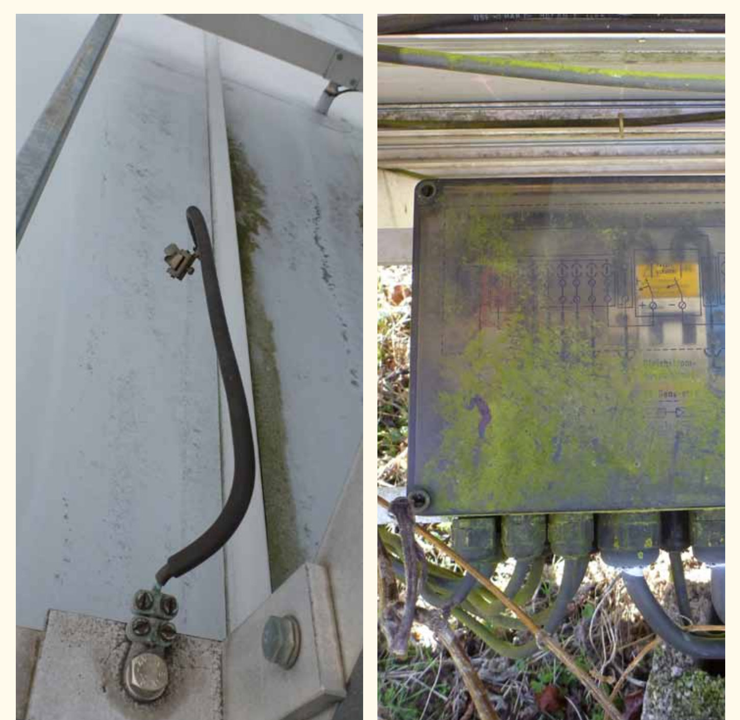
Fig. 9: Earthing wire not properly mounted (Kassel)
