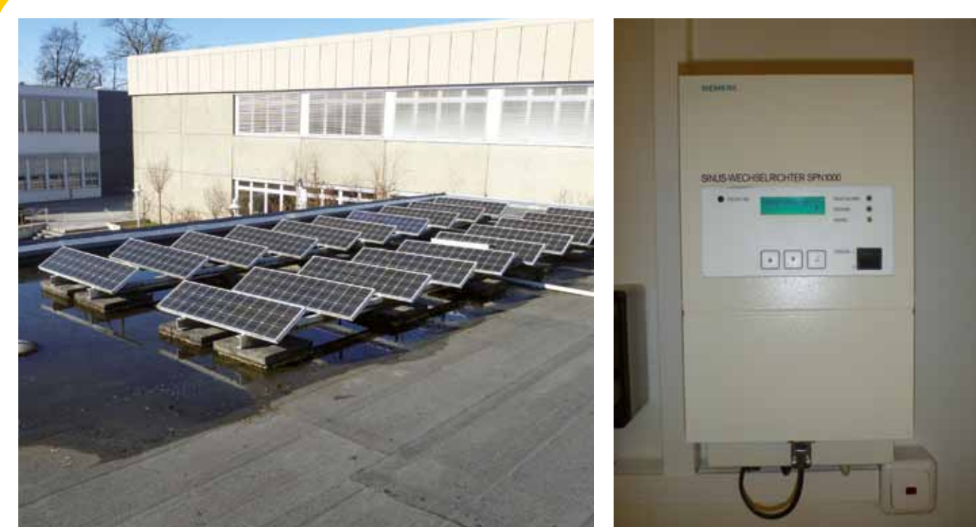
Fig. 2: PV system of nominal power 1.1 kW (20 x Siemens M55) with inverter Siemens SPN 1000 of a grammar school in Coburg in the south of Germany
